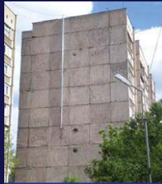
Multi-apartment panel building with exhaust chimney from gas heater installed in one apartment
