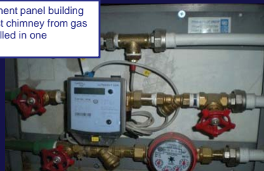
Heat meter installed at the entrance to an apartment in Avan district of Yerevan
