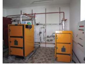
Briquettes fired boiler in the gimnasium from the village Bilicenii Noi, district Singerei. Beneficiaries: 186 persons
