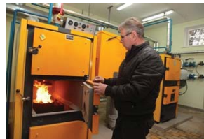
Pellets/briquettes fired boiler in the kindergarten from village Crasnoarmeisocoe, Hincesti district. Beneficiaries: 200 persons
