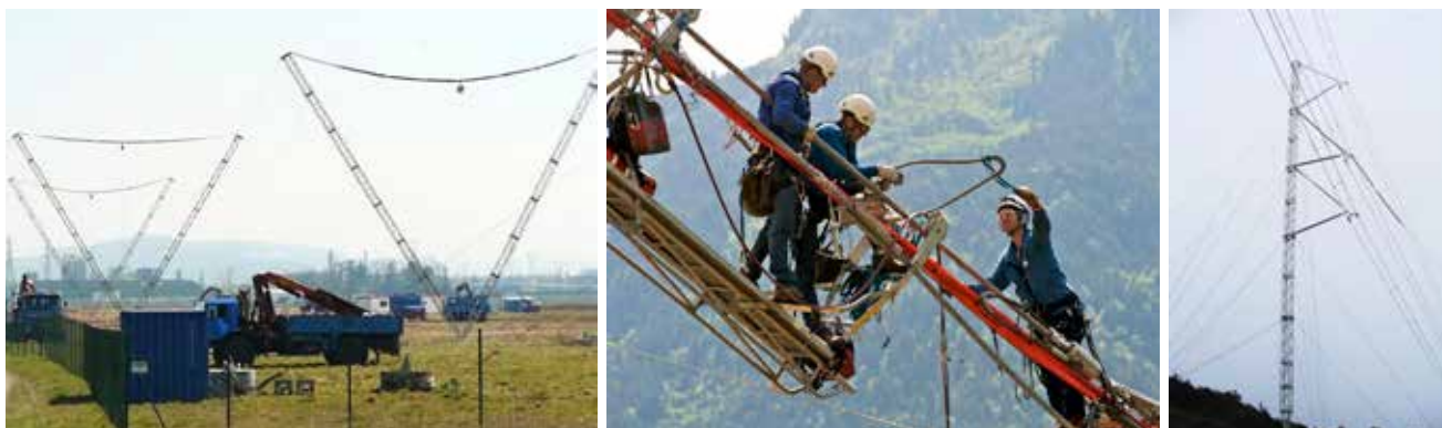
Figure 37: Emergency restoration training and cooperation
