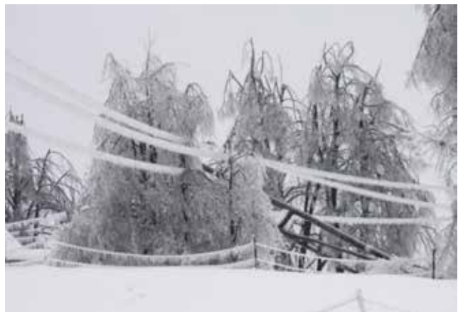
Figure 31. Broken overhead network lines
