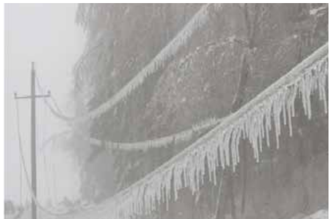
Figure 25. Ice crusts damaging power lines in Carinthia, Austria, in winter 2014
