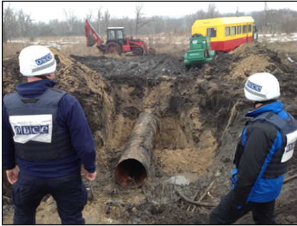
Figure 1: SMM patrol monitoring repair work to a main water pipeline near the Petrivske pumping station in Artema, Luhansk region in January 2017
