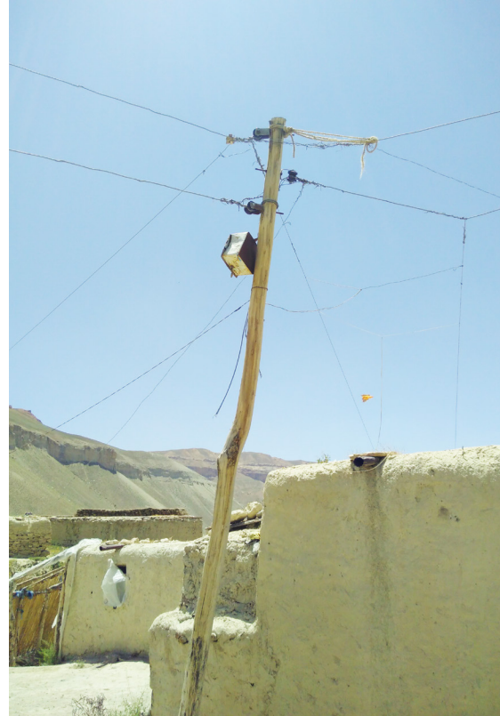
© Zoī Environment Network / Nickolai Denisov, Fatima Akbari Basic infrastructure for power transmission, Bamyan Province, Afghanistan
