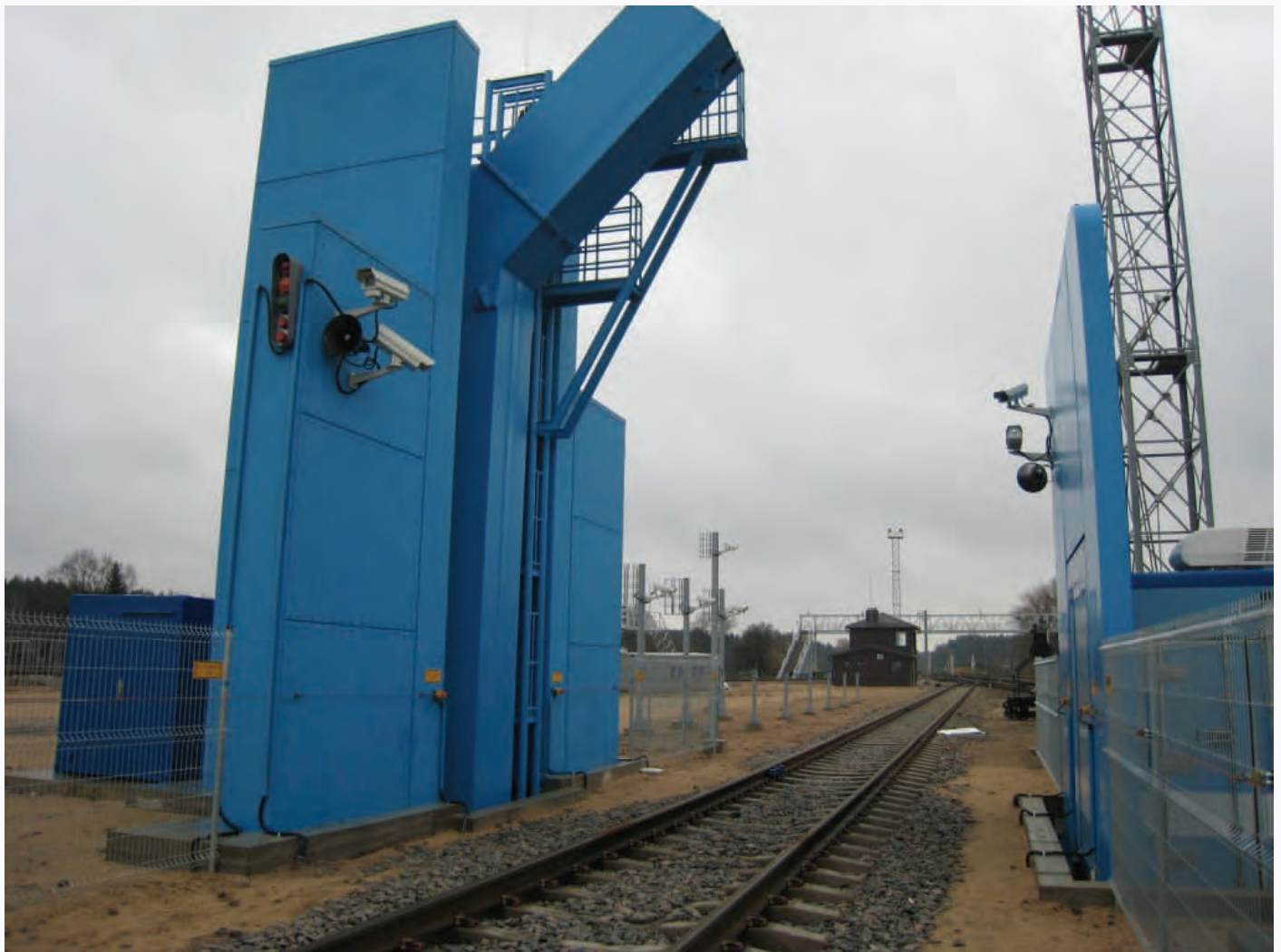
Fixed X-Ray scanner at a railway station , Copyright © UIC
