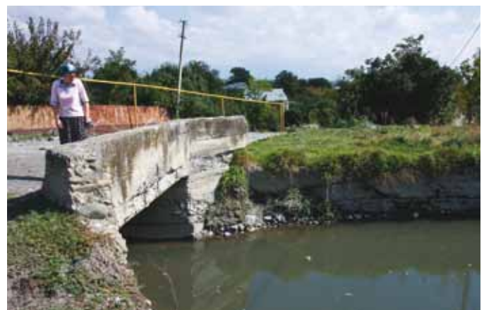
The Nikosi irrigation water project, managed by the CPC, has provided water pumps and pipes to supply river water to the large Saltvisi irrigation channel, for the benefit of farmers affected by the August 2008 conflict in Georgia. June, 2011. (OSCE/Emmanuel Anquetil)
